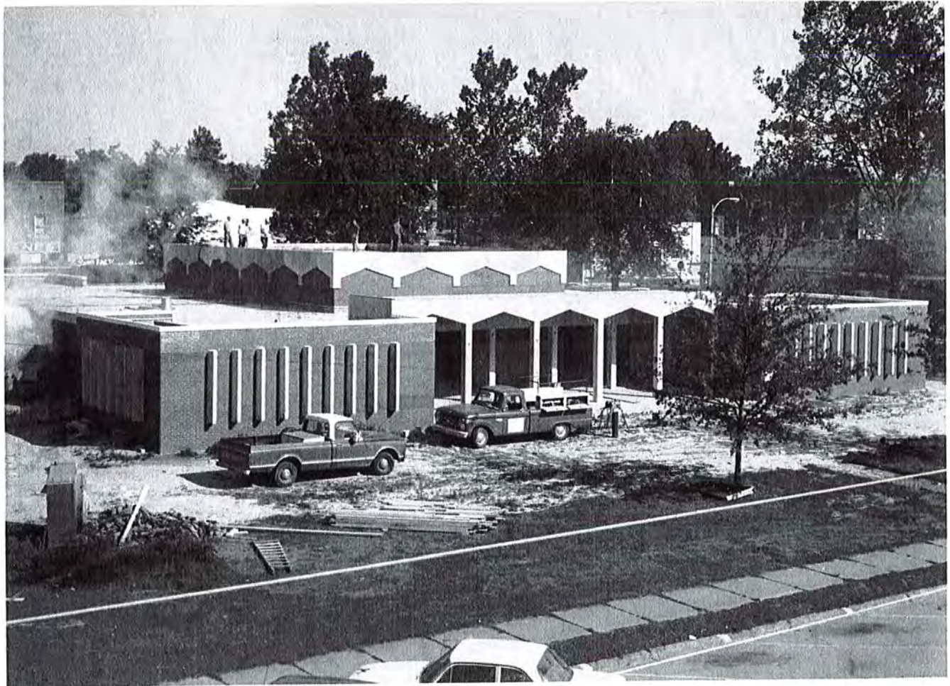
Figure 1: Photograph of the Clay County Courthouse, Eastern District, in the spring of 1967, looking northwest. From the Clay County Times-Democrat . Found at: http://www.cctimesdemocrat.com/gallery/2859 .
